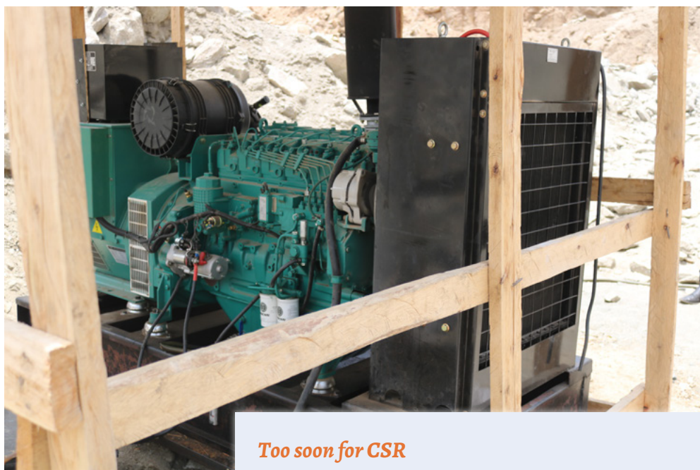
An industrial generator that provides power to the mine site
