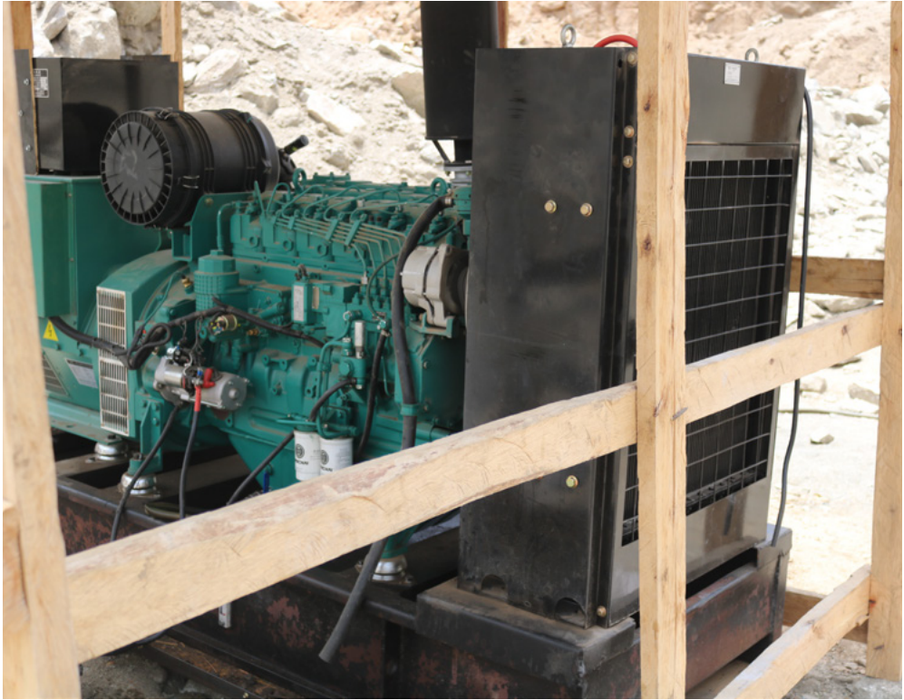
An industrial generator used to supply power to the tunnel
